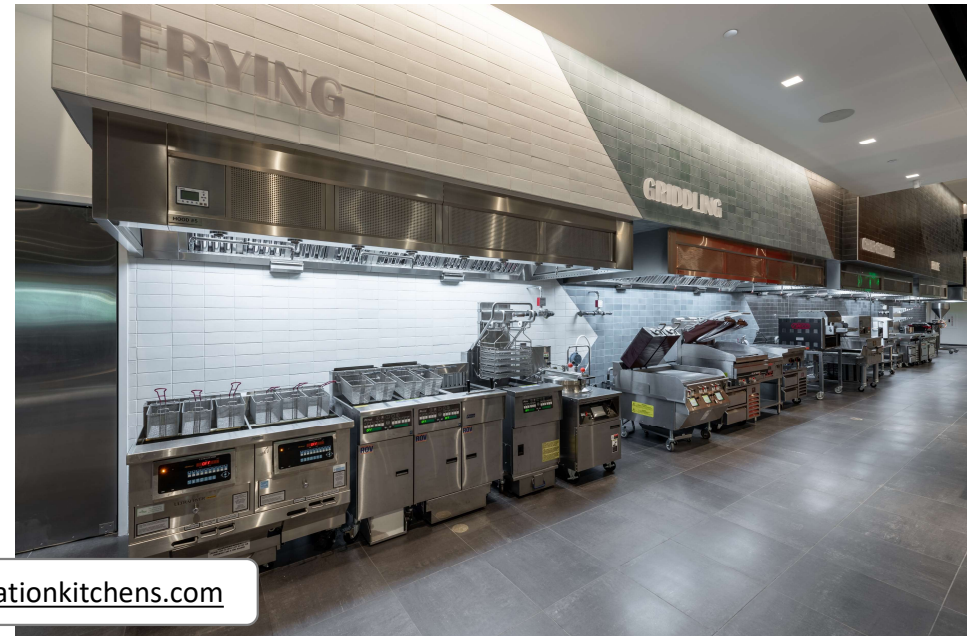
Vignettes - Frying, Griddling, Char-Grilling, and Range are four of the 15 live, fully-functional vignettes at the Middleby Innovation Kitchens.
